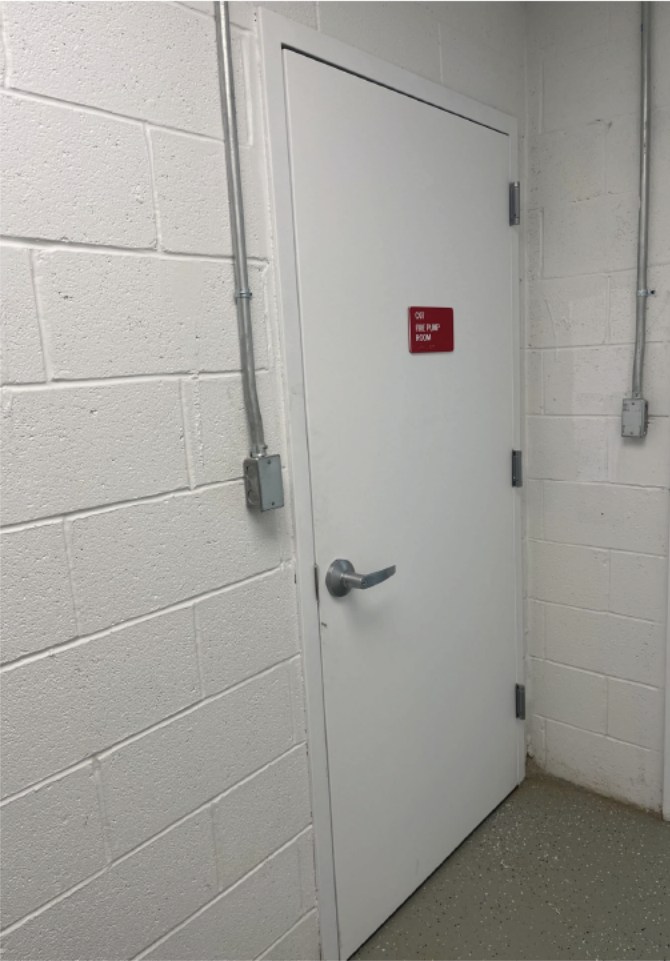
FIRE PUMP ROOM SIGN
